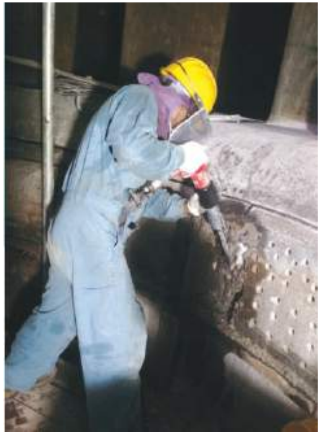
Inside draft tube of Turbine
